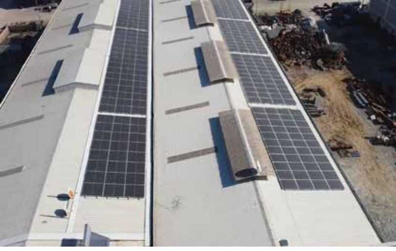
DEHA PLASTİK / ADANA 65 kWp
